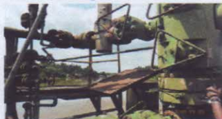
Showing CCU actuator removed.
