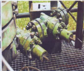
Showing K7L CCU removed & leak point.
